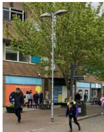
Tower Street lighting 6m light pole
